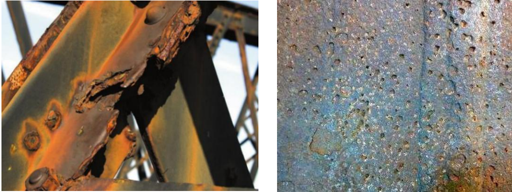
Figure 1.1 : Serious Corrosion of Metals
